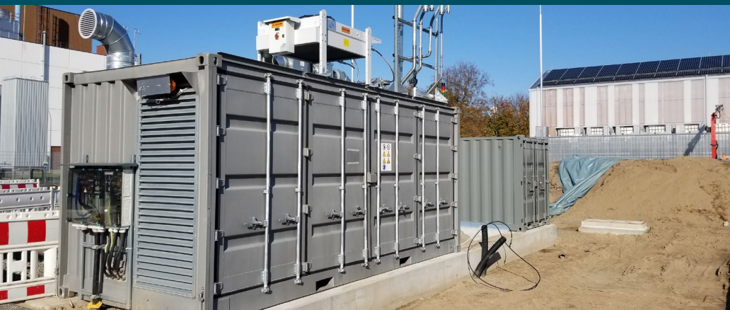
A pressureless solid oxide cell water vapor electrolyzer of 150 kW, which can also be operated in the fuel cell mode, at Energy Lab on KIT's Campus North. Photo: KIT
