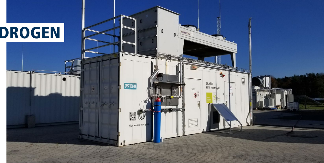
The Silyzer 100 by Siemens Energy is a pressure-driven PEM water electrolyzer installed at KIT's Energy Lab. Photo: IMVT/KIT
